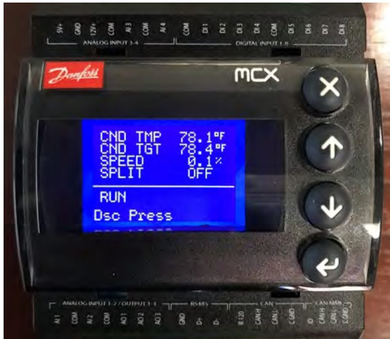
Figure 24 MCX06D CONTROLLER LOCAL DISPLAY
